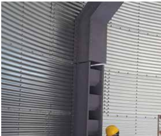
— Photo of bolted sidewall ladders versions
